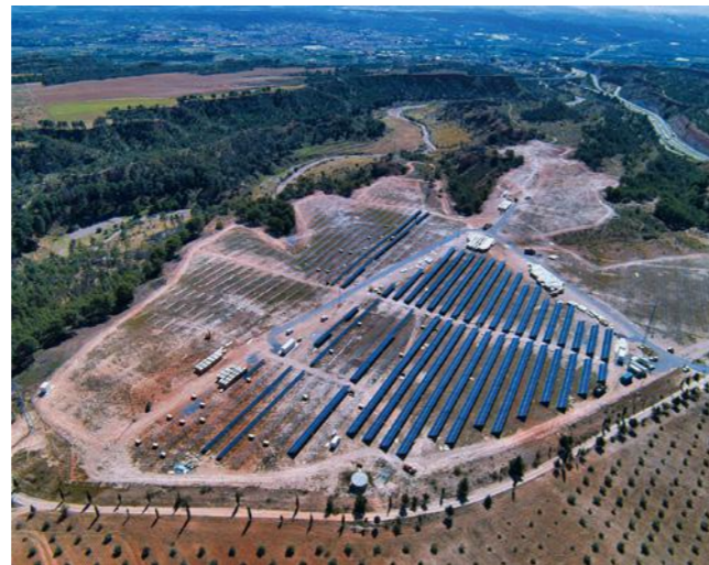
Project name: Solar Power Plant in Sierra Nevada, Spain Project capacity: 7.5 MW
