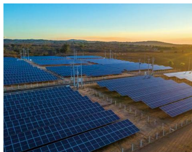
Project name: Setta Solar Power Plant in Pernambuco, Brazil Project capacity: 1.5 MW
