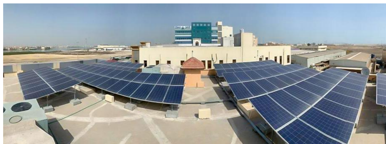
Project name: Rooftop Solar Power Plant of Bahrain Central Bank Project capacity: 40 kW
