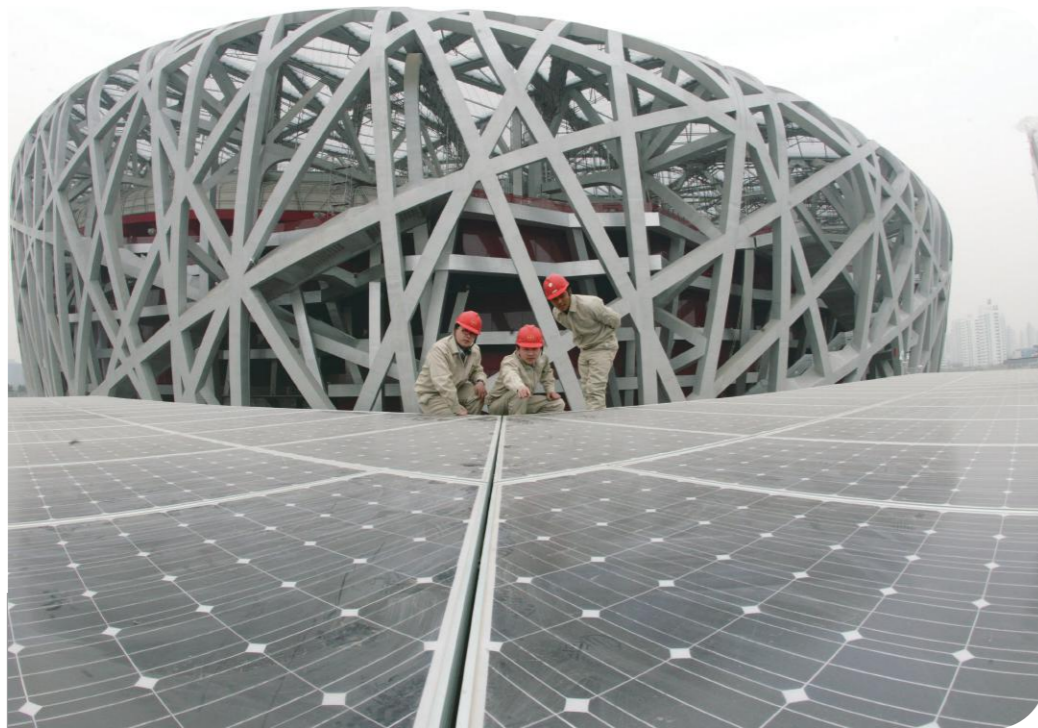
Beijing Bird's Nest Stadium BIPV Project
